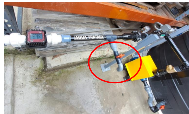
Treated water outlet through a faucet
