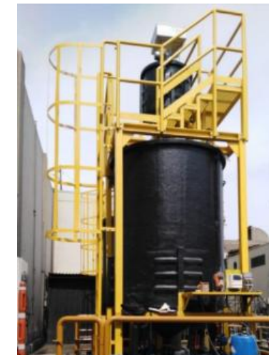
WWTP – Ferreyros Industrial
